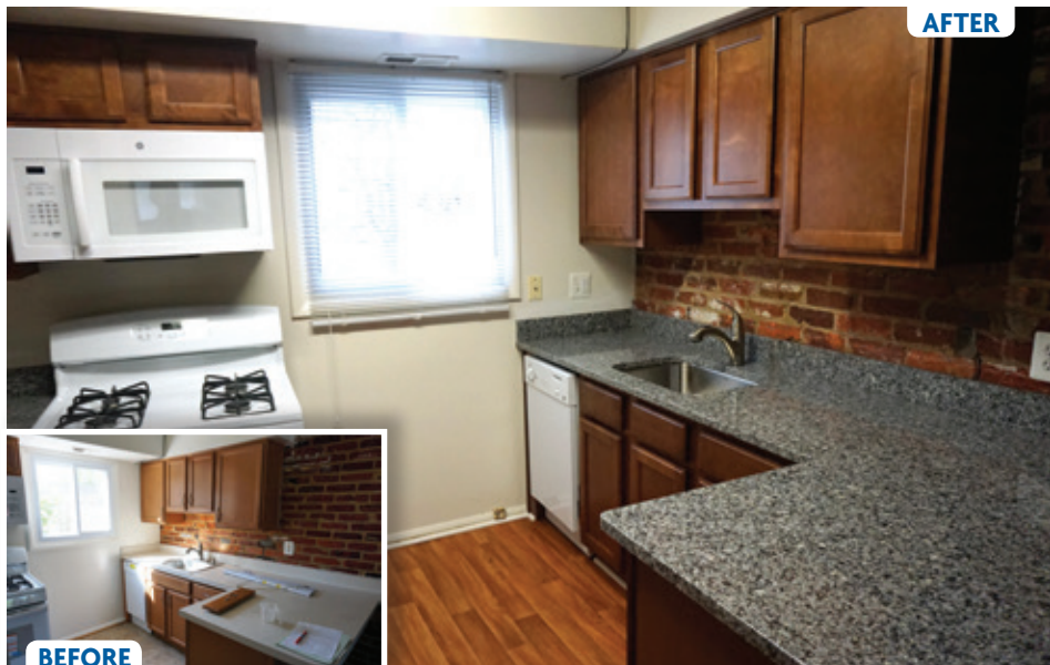
Before and after pictures of a renovated kitchen at St. Margaret of Cortona family residences. All units received the same upgraded flooring, cabinets, countertops, and fixtures.
